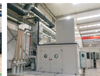
Automatic recovery type sandblasting room
